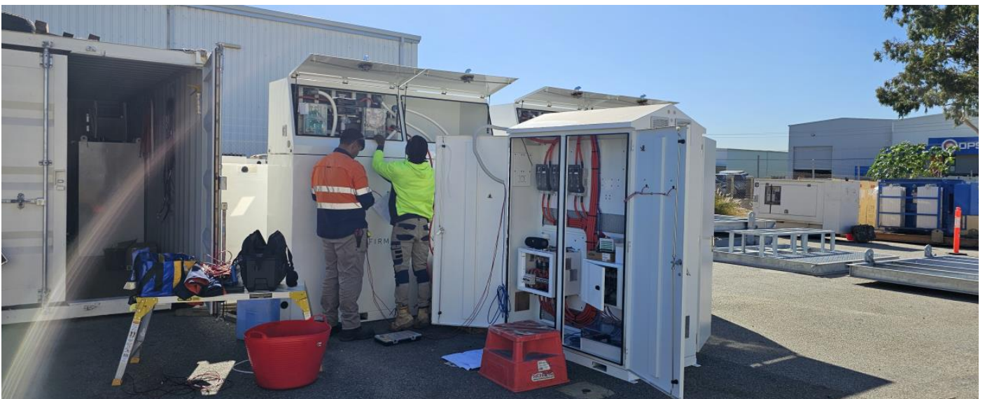
The electrical team from SMEC Power and Technology completing and commissioning battery models and control system for the next microgrid project.
