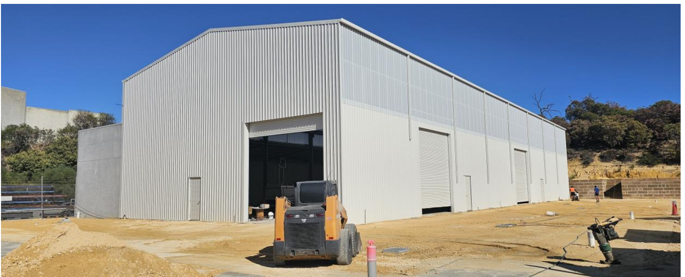
Thorion Energy flow partner SMEC Power and Technology building the new electrical workshop increasing the floor area to 4000 square meters.
